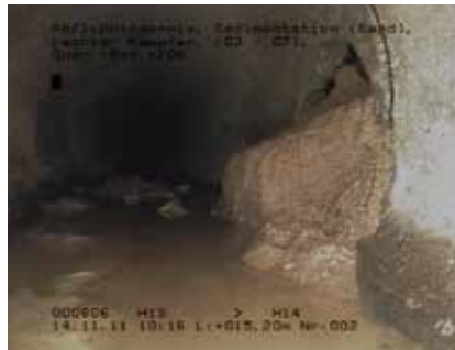
Damage before the rehabilitation
